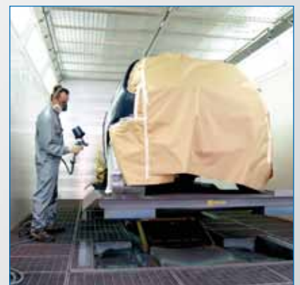
The lift HLS as in-ground installation in the spray booth.
